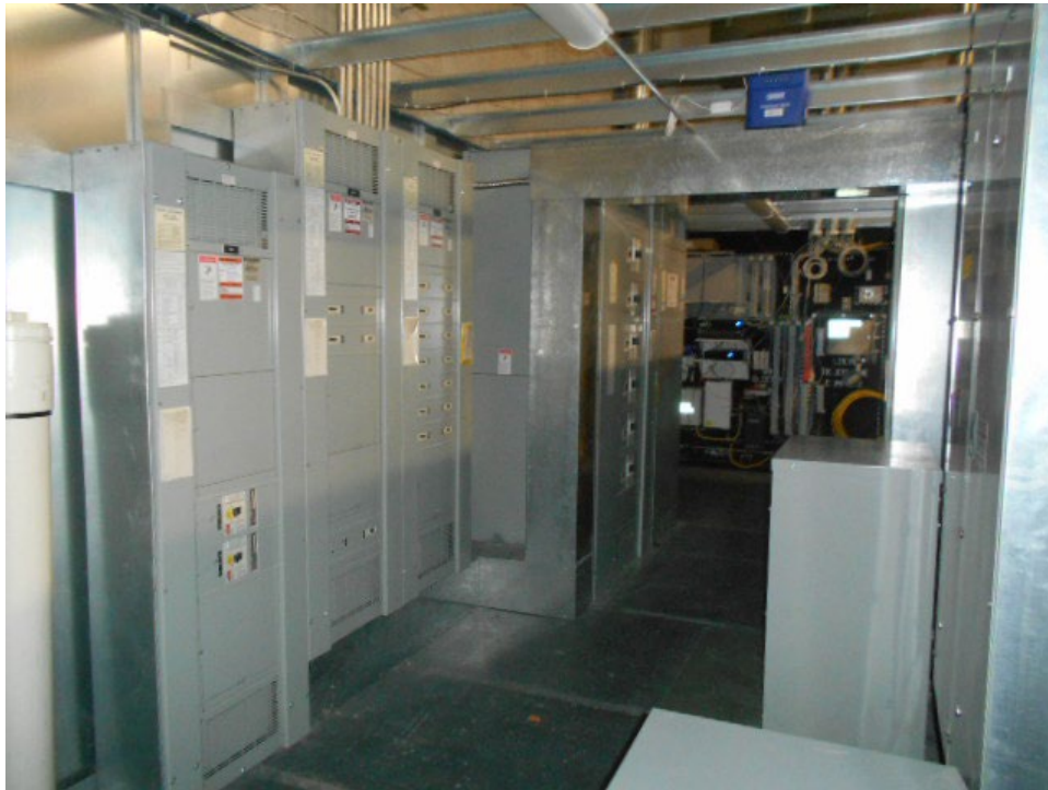
Electrical Service Room
