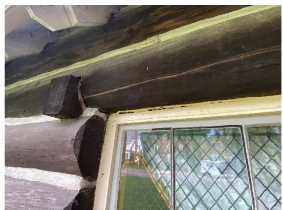
Exterior window caulking needs repairs
