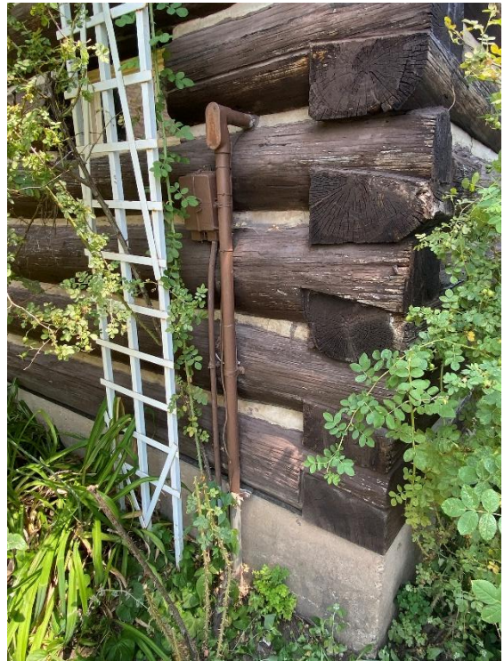
Trellis electrical feed
