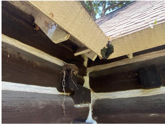
Gutters in poor shape and bird's nest
