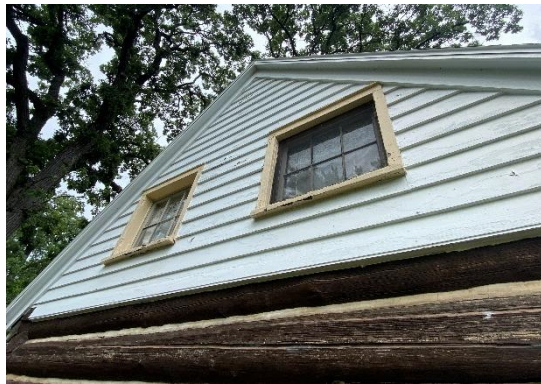
Gable siding needs to be repainted
