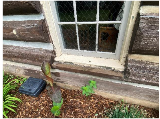
Repairs to the exterior windowsill needed
