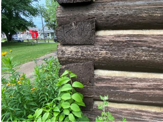
Repairs needed at the end of logs
