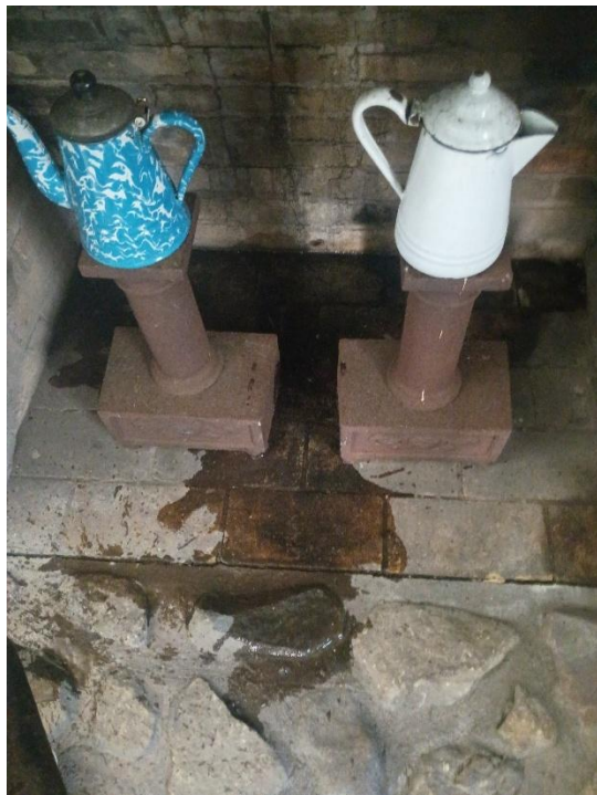
Chimney needs repairs to prevent leaking
