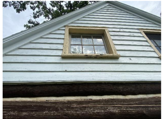
Siding paint and chinking needs attention
