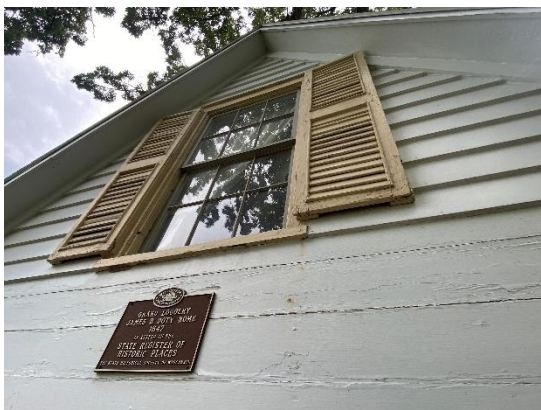
Siding and shutters on the north side need repairs
