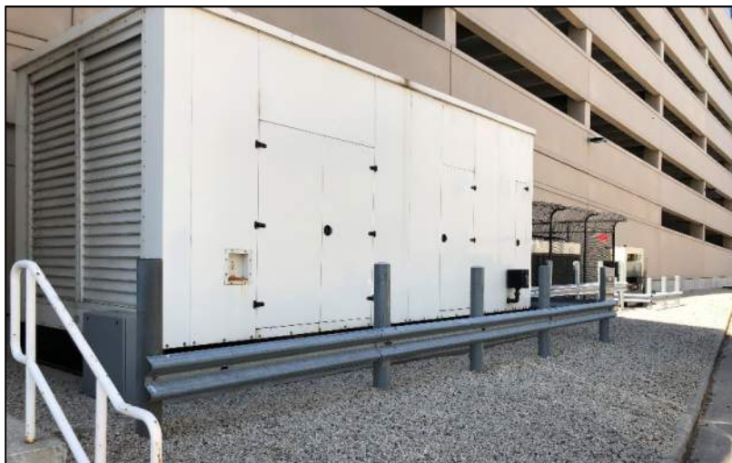
Figure 7: Three existing electrical or server boxes on northeast corner of parking ramp
